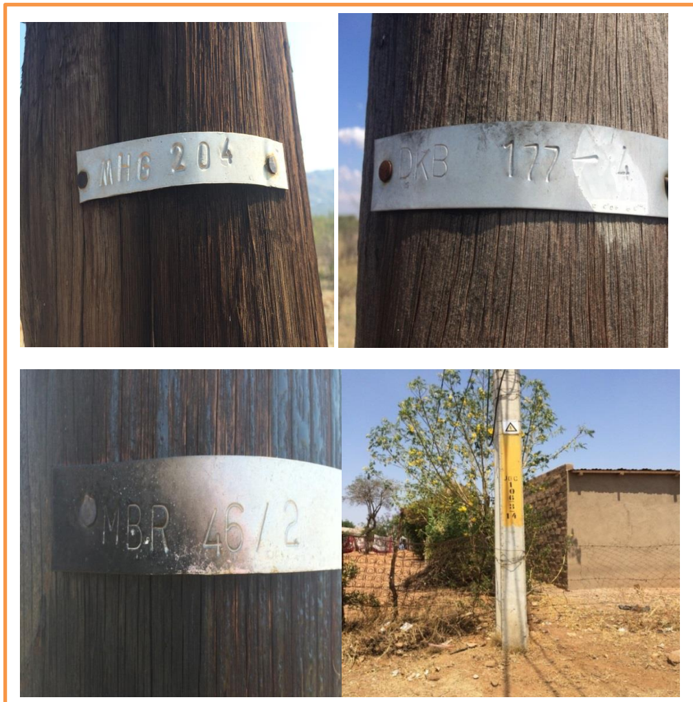
Figure 4.1: Labels on poles mounted with transformers (Rampjapedi, 2015)
