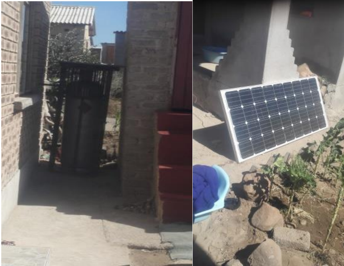
Fig 5.6 (left) Gas cylinder used for the gas stove and freezer in Victoria Ranch (right) Solar Panel used to charge batteries for lights in Victoria Ranch. (Source: Author's own photograph, August 2016)
