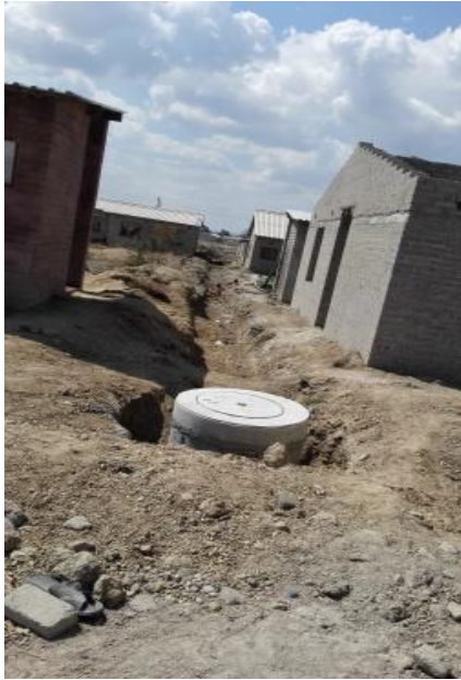
Fig 5.4 Sewerage Trench in Victoria Ranch where the destruction happened (Source: Author's Own Photograph, August 2016)
