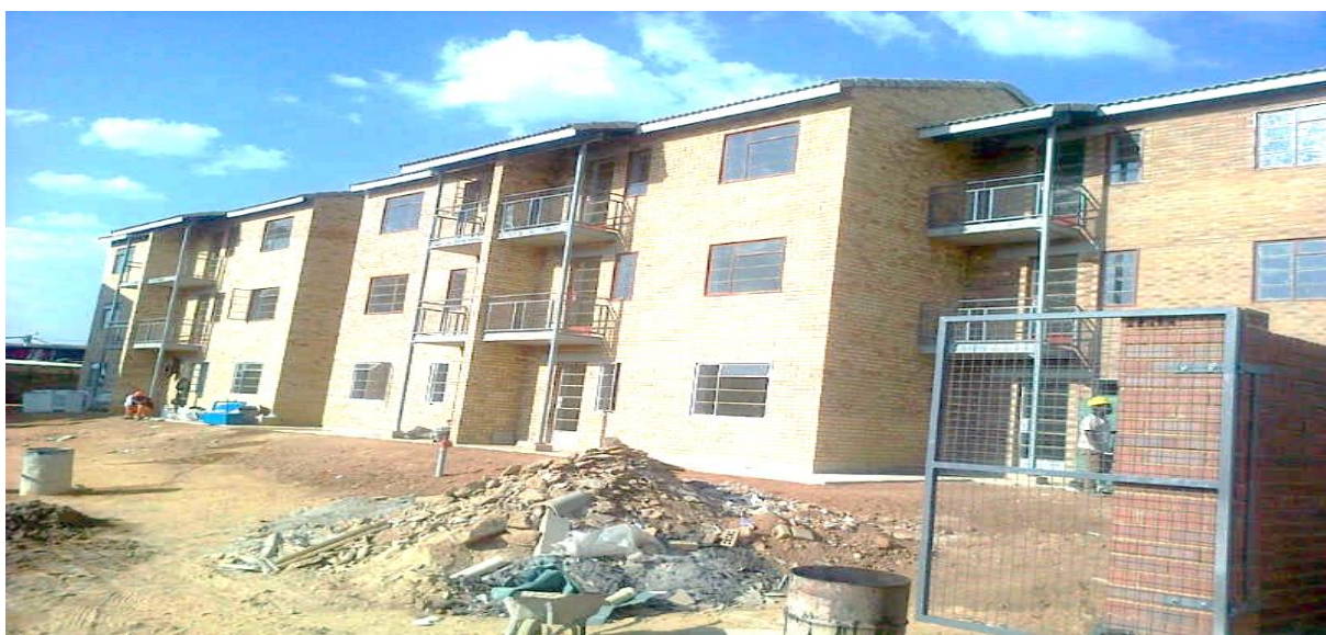
One of the blocks of the FLISP housing project under construction in 2016. Source: Own.
