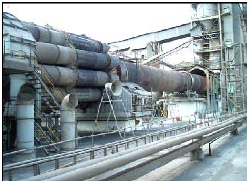
Figure 2-2: Long dry kiln (as cited in the PPC Background document for the Proposed Secondary Materials Co-Processing Programme, 2006, pg 5).
