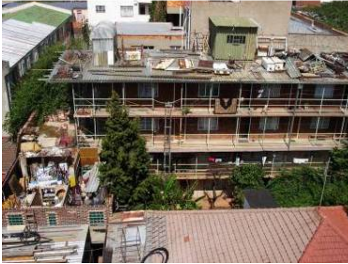
Figure 22: Poorly maintained high-rise building in Yeoville
