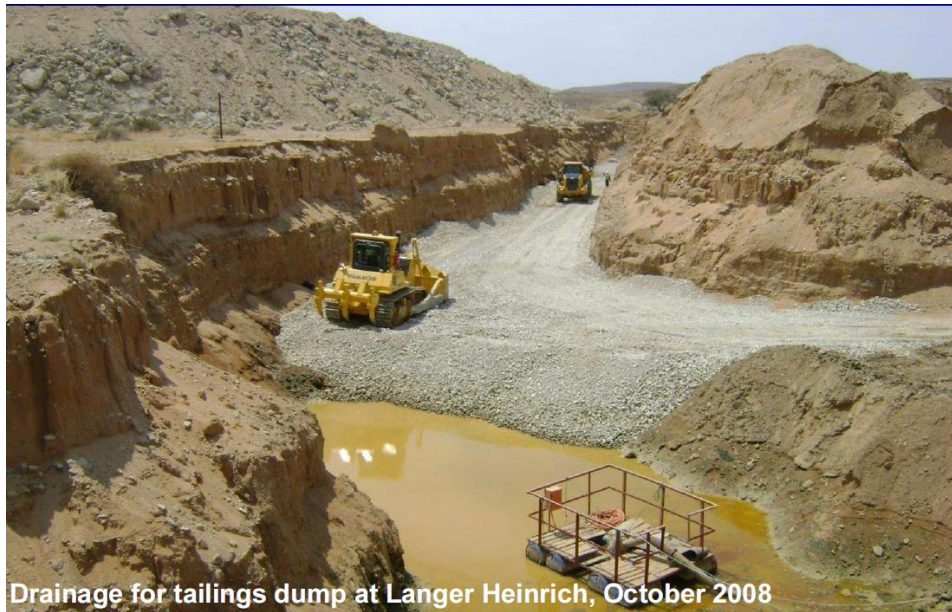
Figure 1. The seepage from the tailings dump at Langerheinrich in 2008 (Source: www.iaea.org/OurWork/ST/NE/NEFW/documents )
