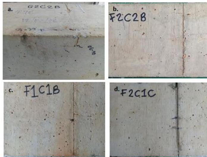
Figure 4.27: Corrosion-induced cracks of concrete with reinforcement at (a & b) edge (-E), and (c & d) middle of beam (-M).
