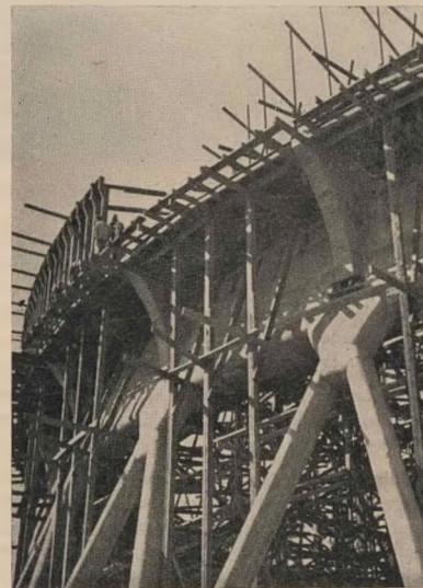
9. Detail showing the tops of legs, the brackets and shuttering for the annular duct.
