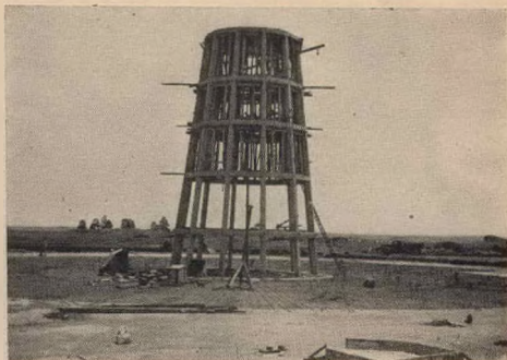
4. The central structure in reinforced concrete, which carries the red-wood stacks and spray piping, with the reinforcement for the pond bottom.
