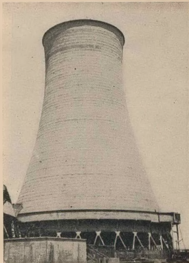
12. The completed shell. The striations on the surface mark the progressive stages of concreting in consecutive rings 4 feet high.
