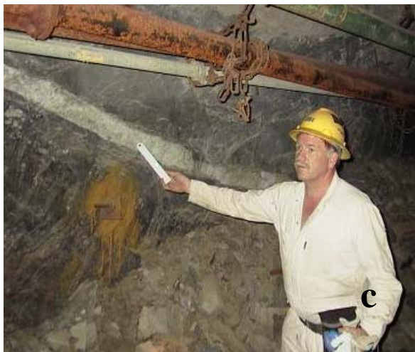
Figure 1.4 Large wedge collapse (a) with vertical jointing (b) and bounded on the upper side by a prominent flat dipping vein (c)
