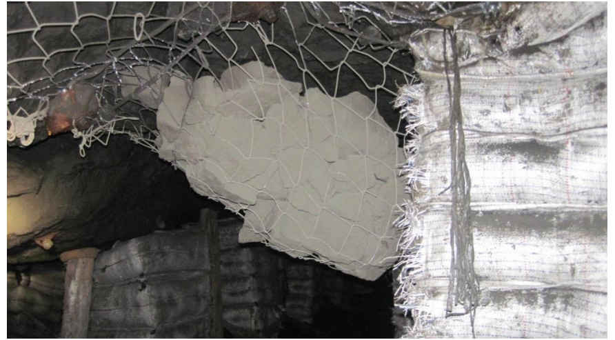
Figure A- 24: Chain link mesh retaining broken hanging.
