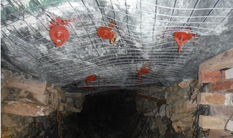
Figure A- 13: Good weld mesh condition in a gully and hydrabолts
