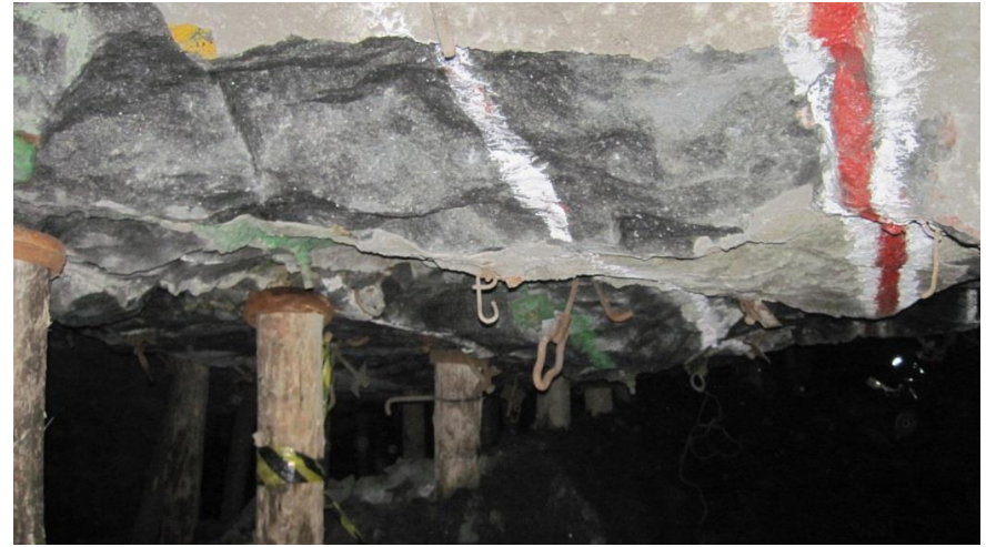
Figure A- 31: TSL damage due to large block.
