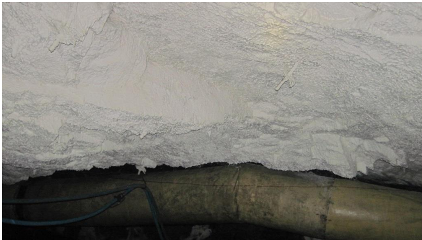
Figure A- 27: Rock mass condition after TSL application.
