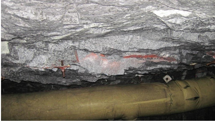
Figure A- 26: Rock mass condition at pothole edge.
