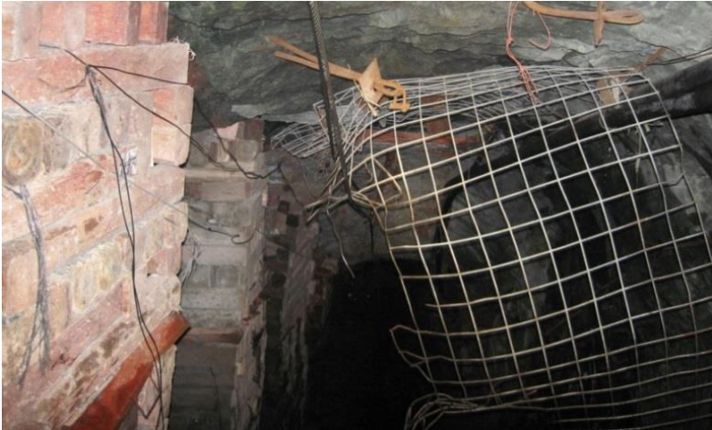
Figure A- 17: Weld mesh damage caused by scrapers
