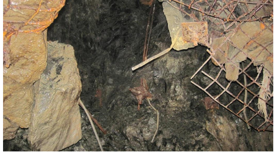
Figure A- 21: Heavily rusted mesh connected to anchors by s - hooks
