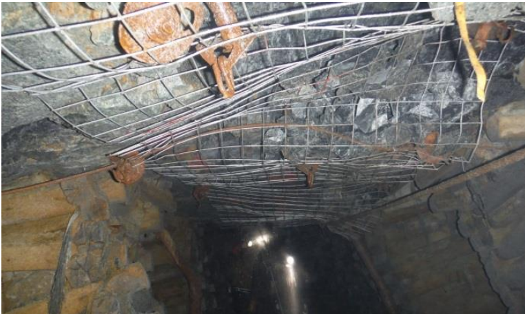
Figure A- 14: Weld mesh retaining broken rock
