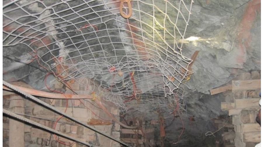
Figure A- 18: Weld mesh damage caused by blasting
