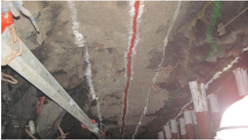
Figure A- 29: TSL condition in gully.
