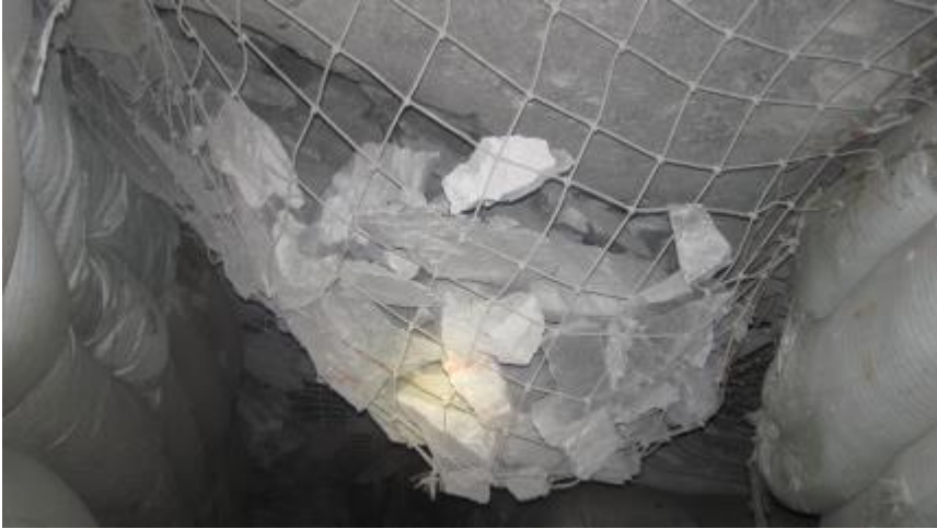
Figure A- 6: Net retaining broken hanging without rock bolts
