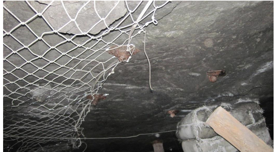
Figure A- 25: Blasted-on mesh with steel rope to absorb blast impact
