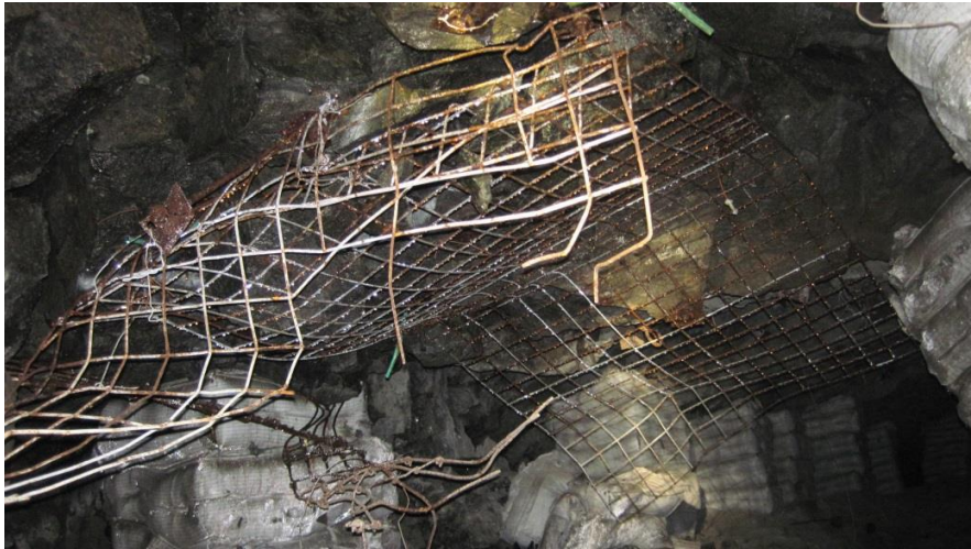
Figure A- 20: Scraper damaged mesh
