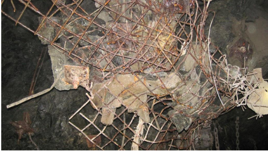
Figure A- 19: Blast damaged mesh still retaining rock
