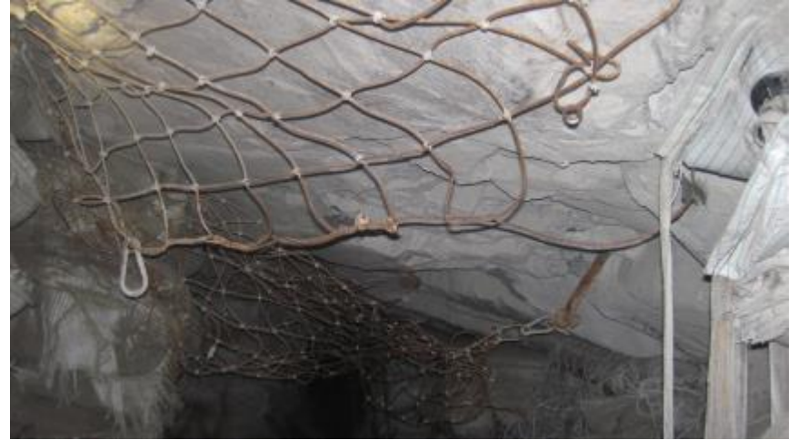
Figure A- 8: Failed and rusted net in back areas
