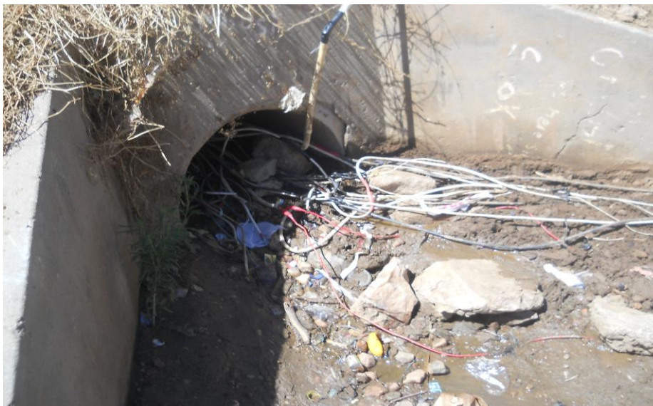
Photo No. 21: Illegal Power Supply in Windhoek 608
