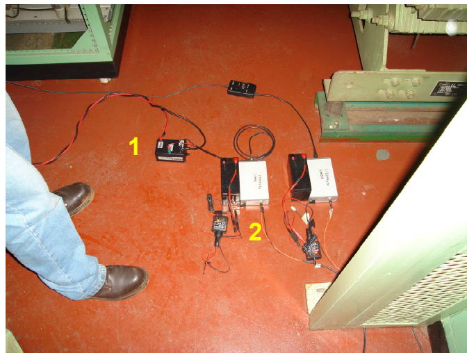
Figure 5.2.3 – The fibre optic setup for the sub station where the yellow numbers indicate the various components used
