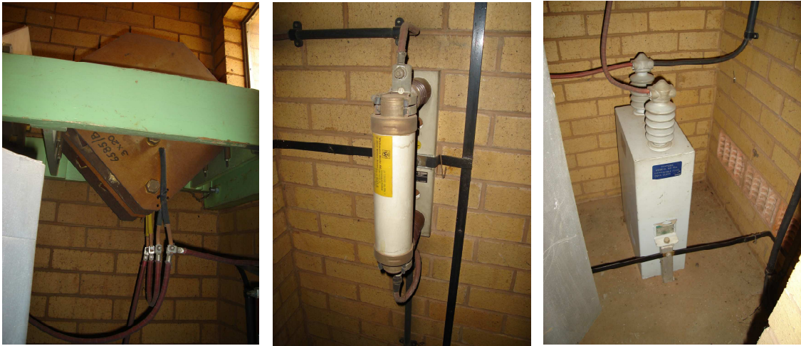
Figure 5.2.5 – The components that make up the harmonic filter, the photo on the left is the inductors, the middle photo is the series fuse and the photo on the right is the capacitor
