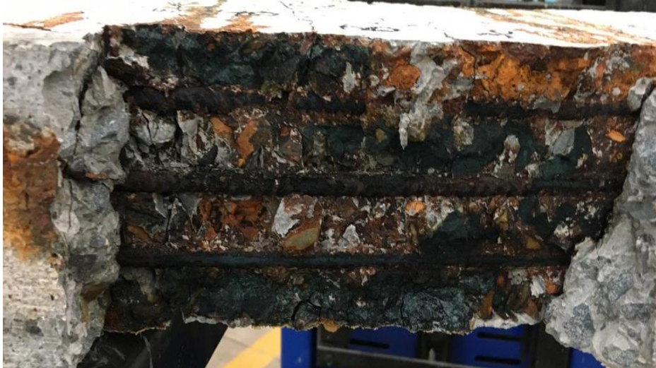
Figure 3. 9: Photograph showing corrosion products
