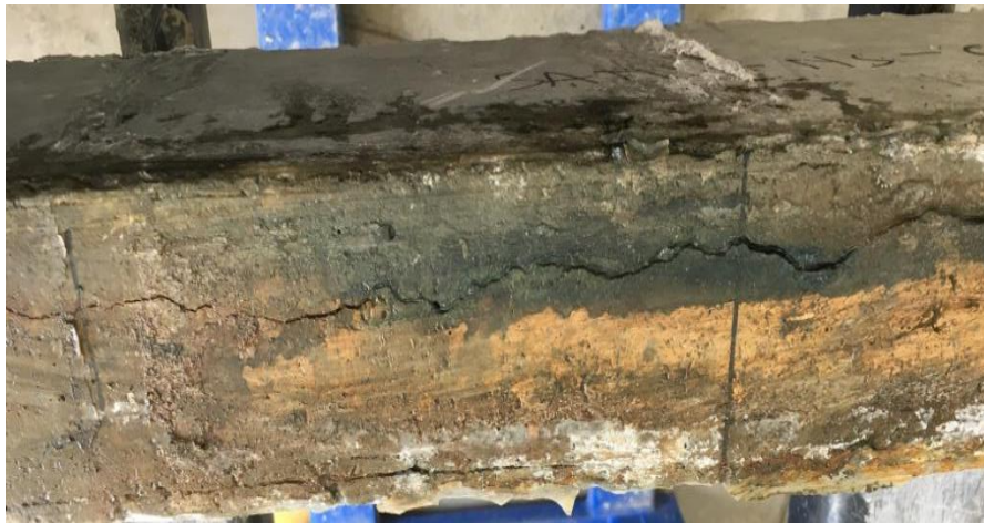
Figure 3. 8: Photograph showing longitudinal cracks on concrete surface
