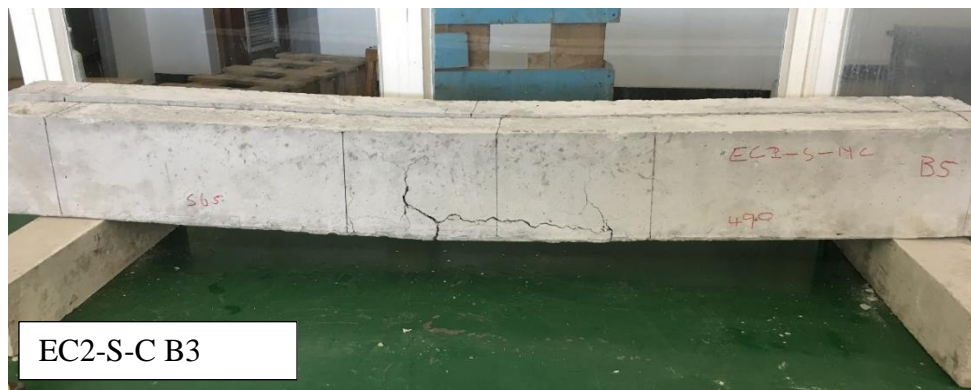
Figure 4. 13: Flexural crack pattern developed on EC2-S-NC beams
