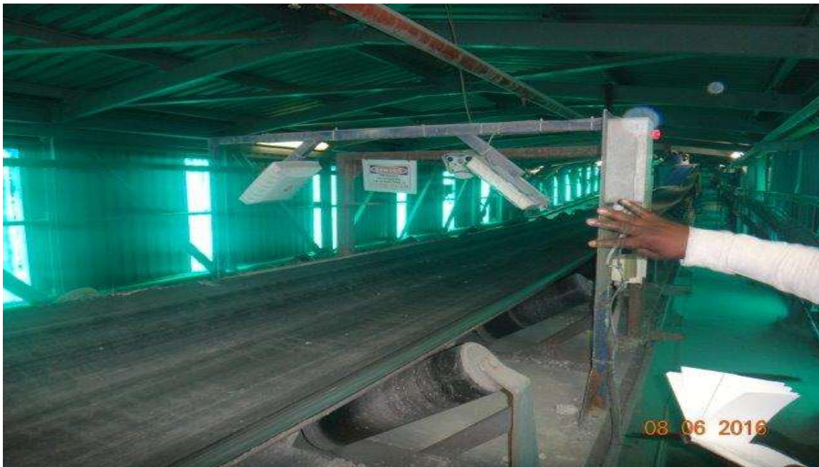
Figure 3.2 Equipment used to detect the RFID tags on the belt to plant (Doornkop Shaft, 2016)
