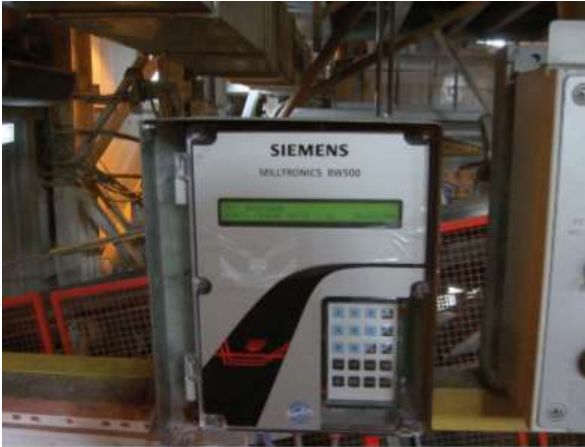
Figure 2.3 Electric weightometer for tonnage (Doornkop Shaft, 2017)
