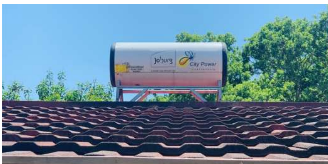
Figure 4.6 An example of a Solar Water Heater provided by City Power. Source: Authors Own, 2020
