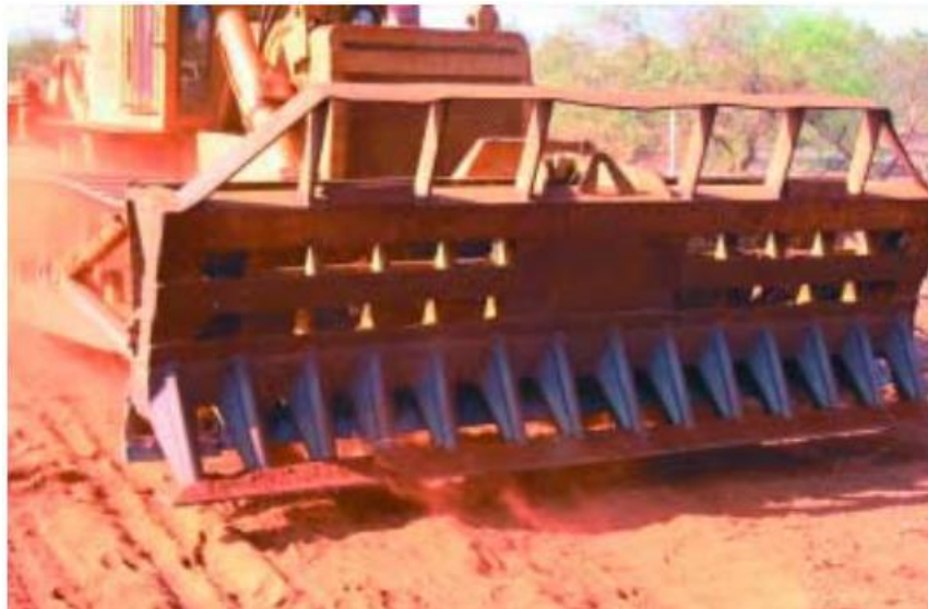
Figure 2.2 Mechanical control methods employed in Kassala through the use of bulldozers (Department of Natural Resources and Mines (Sudan), 2003)
