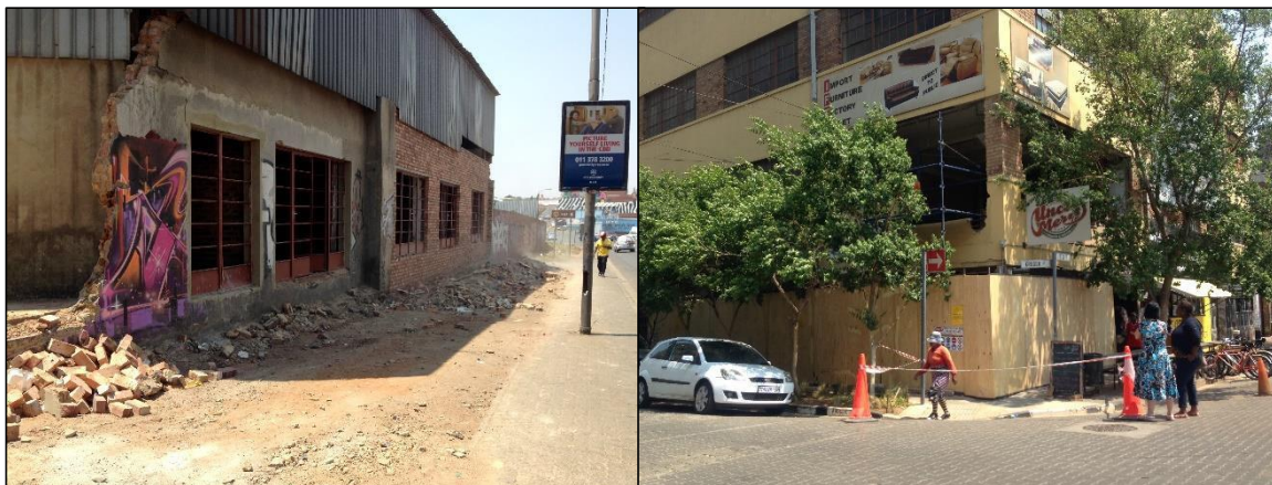
Figure 25: Left: Windows and doors being knocked out for new Market Up development, opening up onto Albertina Sisulu Road. Right: Windows being knocked out onto the corner of Fox and Kruger Street for new Propertuity Sales office. (Source: Rory Murtagh 2015)
