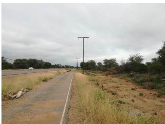
Photo 5: Installation of power lines incomplete
