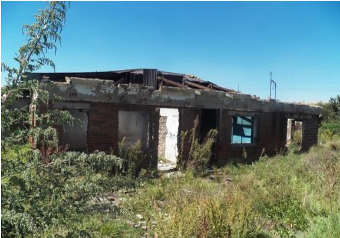
Figure 5.2: A collapsing house near the Klip River in Freedom Charter (Source: Mpho Nenweli, March 2013) (A part of this house was occupied at the time of my fieldwork)
