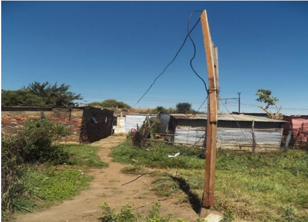
Figure 7.1: Illegal electricity connection in Freedom Charter (Source, Mpho Nenweli, March 2013)
