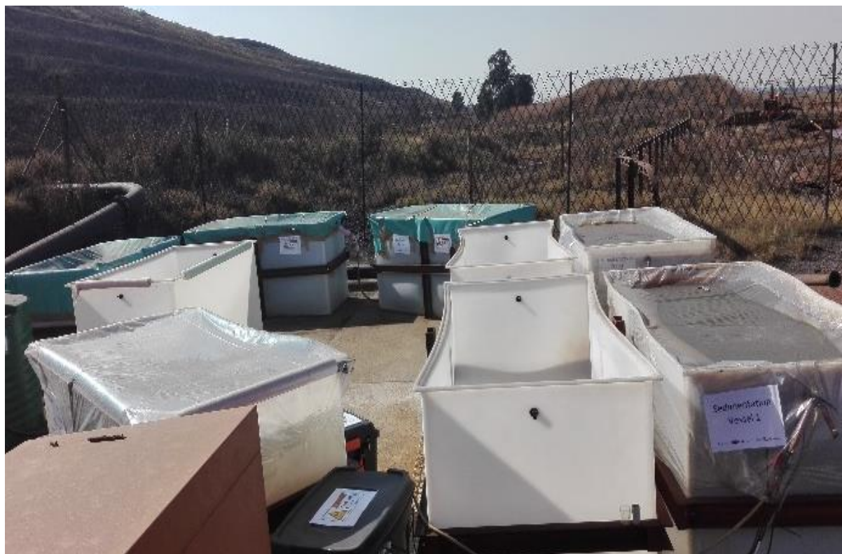
Figure 10-4: AMD remediation pilot plant at mine dam site (photographs taken by authors)
