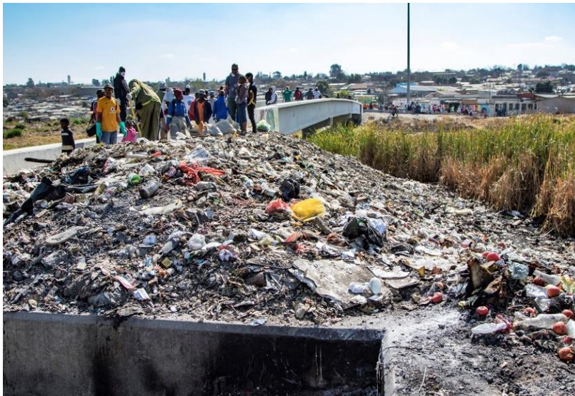
Figure 4.16: Solid waste heap constricting a water course
