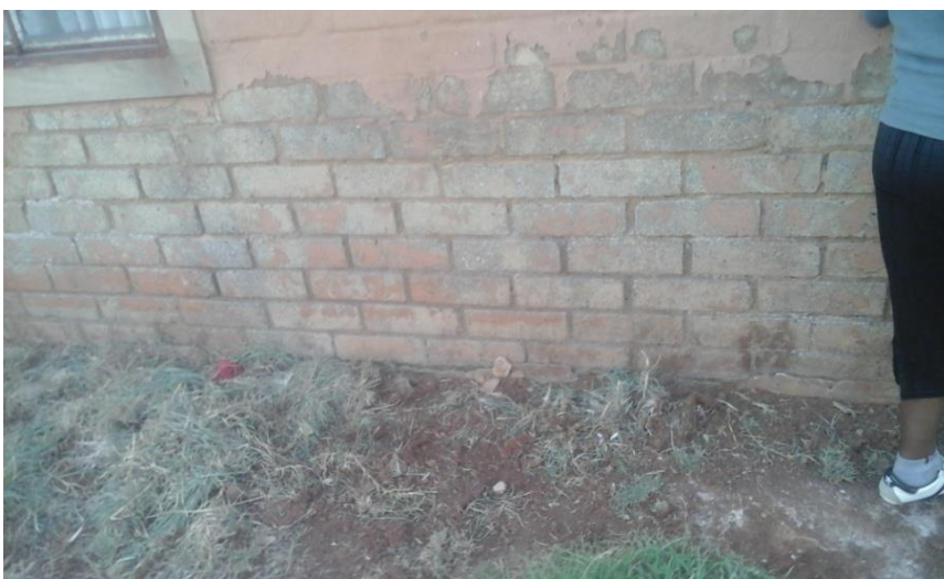
Figure 11: Flood damage to houses in Bramfischerville
