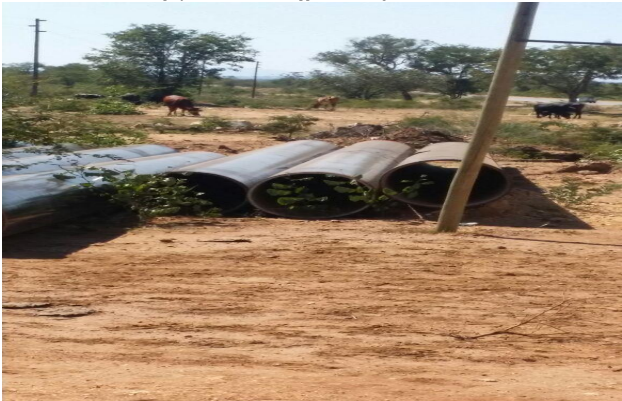
. Picture 1: Nandoni to GLM project- Construction stopped due to litigation
