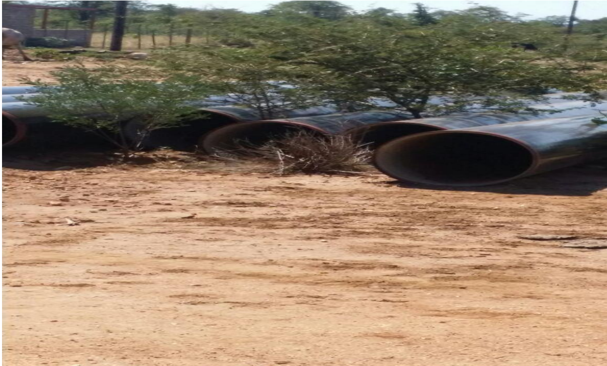
Picture 2: Nandoni to Giyani pipeline project: some of the pipes awaiting installation. The lengths of delays due to court litigation are evident as trees have grown in between the pipes.
