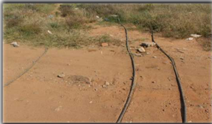
Figure 13: - Illegal electricity cables in Zamimpilo. Source: Janice Beckett, Soweto Urban News 2018
