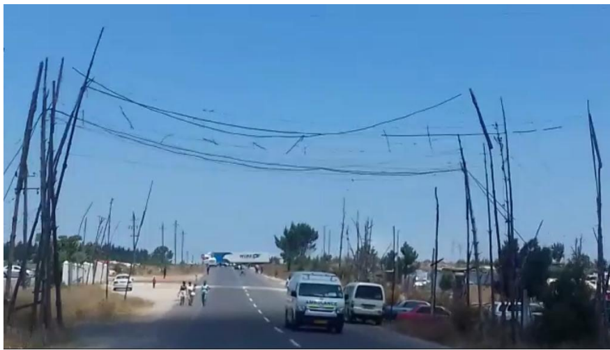
Figure 1: Izinyoga-Nyoga - illegal electricity connections
