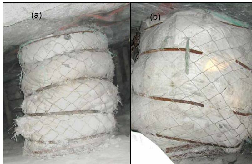
Figure 4.21 Two mesh packs installed in a stope (a) soon after installation and (b) with lateral dilation and strap failure
