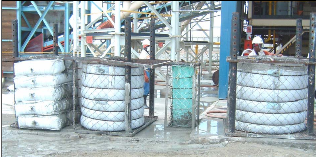
Figure 3.1 The frame at Karee 3 Shaft grout plant where the packs were cast
