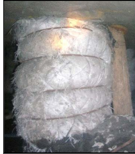
Figure 4.11 A 750 mm diameter RSS pack installed at Spud shaft with 150 mm closure
