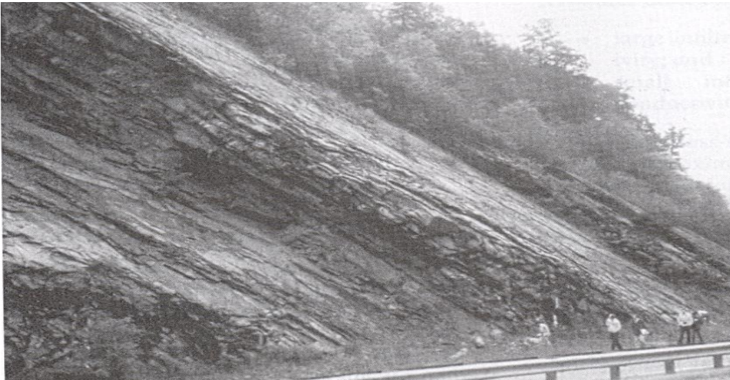
Figure 6: Planar failure on smooth, persistent bedding planes in shale (Interstate 40, near Newport, Tennessee), after Wyllie and Mah, 2004
