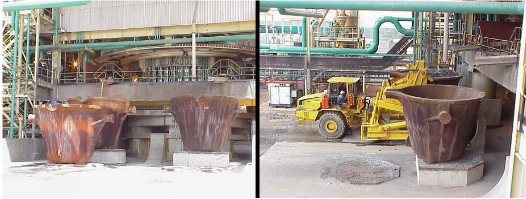
Figure 2.16 Slag-tapping end of the Chambishi 40 MW furnace
