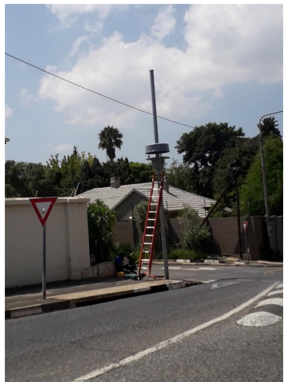
Figure 2: An example of the new Artificial Intelligence CCTV camera infrastructure, called 'Vumacams', being installed, Manoim 2020
