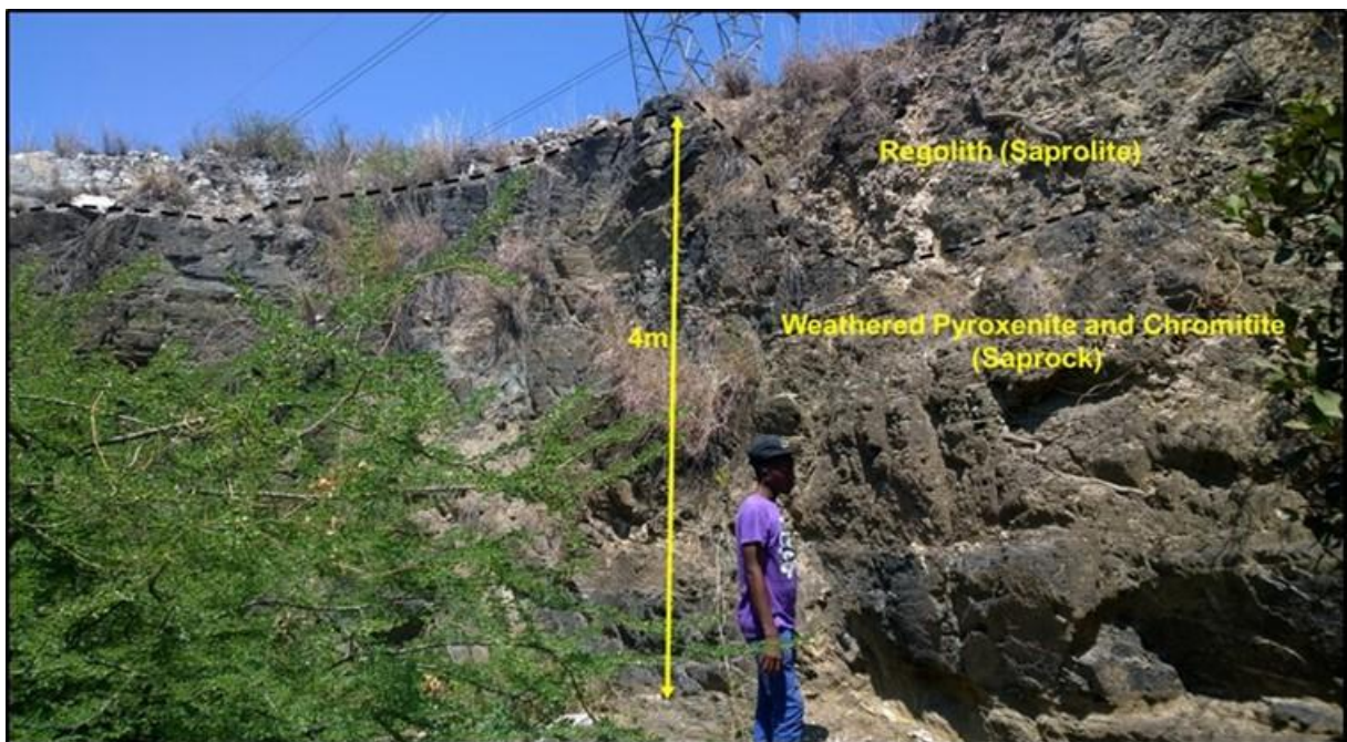
Figure 28: A trench showing the regolith and weathered aquifers in the Tweefontein farm.
