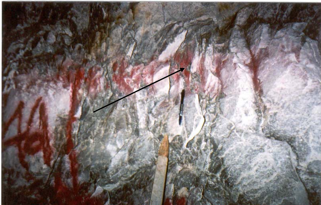
Figure 3.5a Stress induced fractures in a development end
