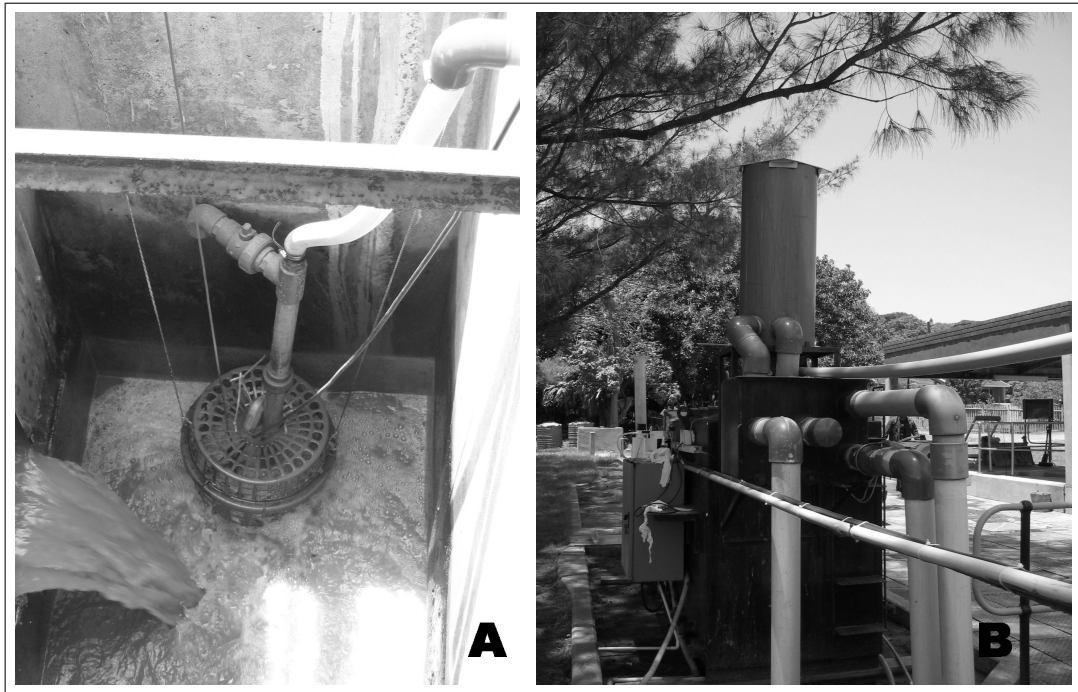
Figure 3.1: (a) A photograph of the pump used to feed wastewater to the ABR and (b) The feed and overflow pipes, and the splitter box above.
