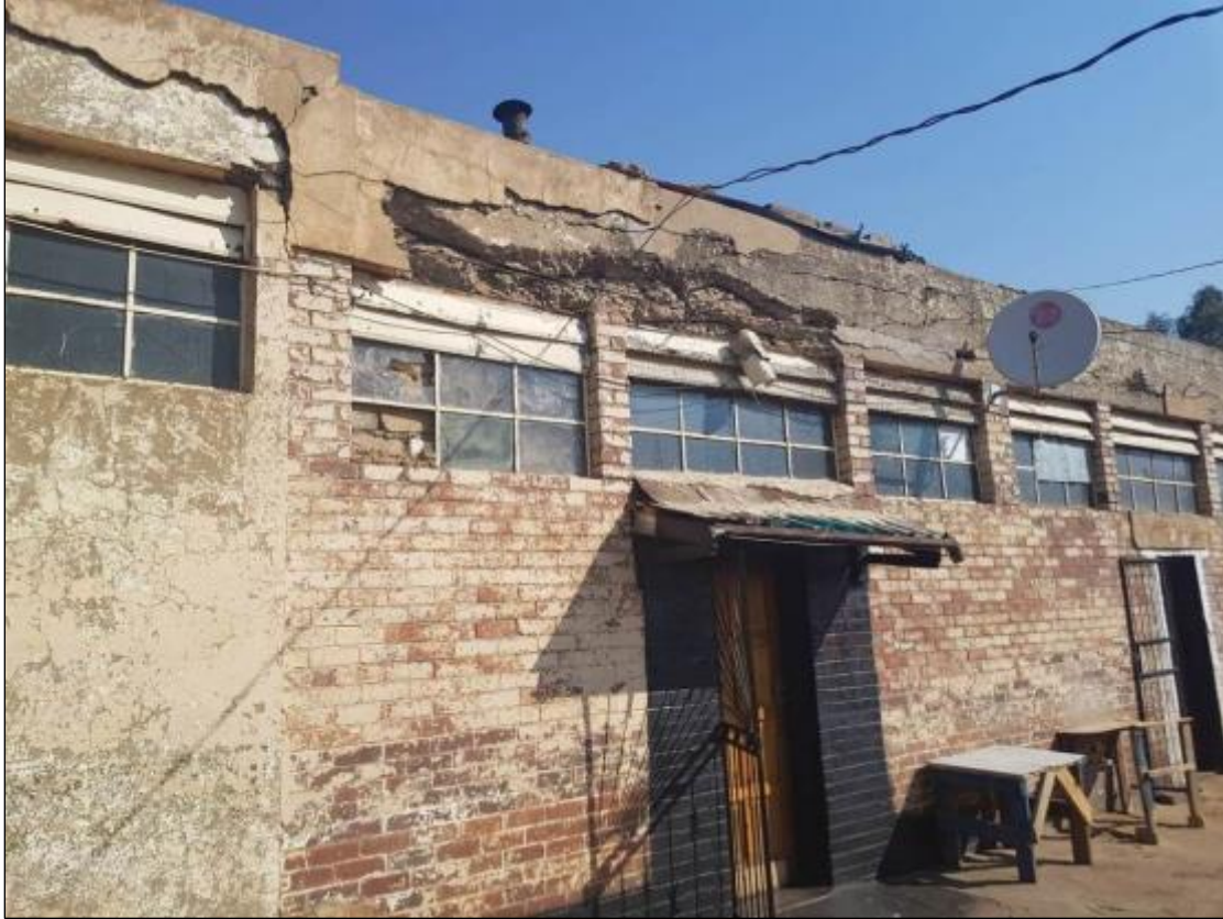
Figure 3.14 The former mine hostel building at Bottom Compound has been declared structurally unsound but is still occupied. (Author's photograph, 18 August 2021)
