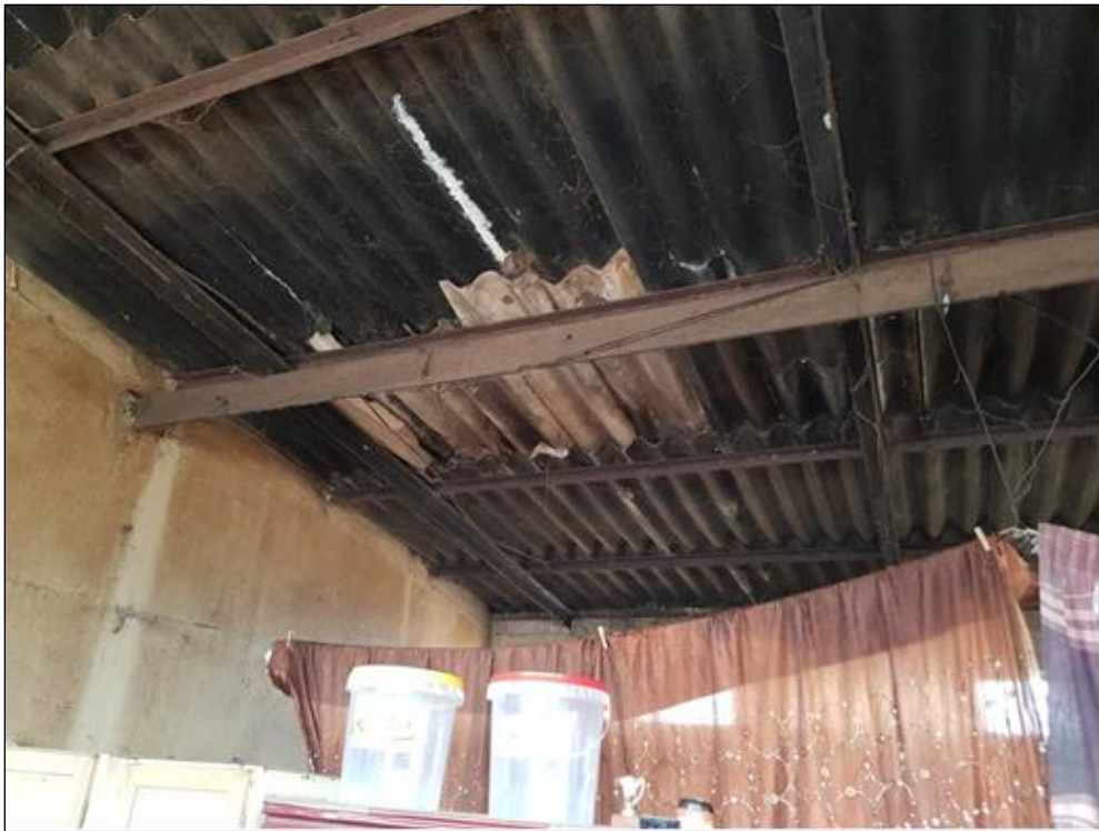
Figure 4.4 Buckets are used to collect rain water from a leaking roof at Bottom Compound. (Author's photograph, 1 October 2021)
