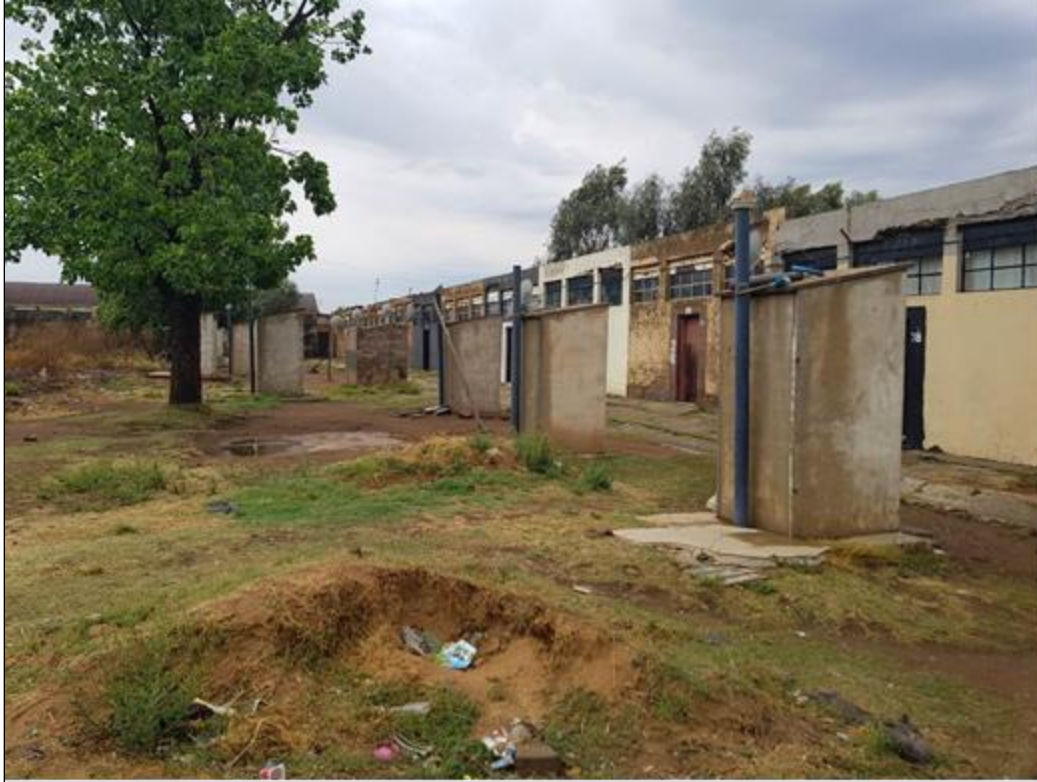
Figure 4.2 Aging temporary infrastructure at Bottom Compound is inadequate for the community. (Author's photograph, 1 October 2021)
