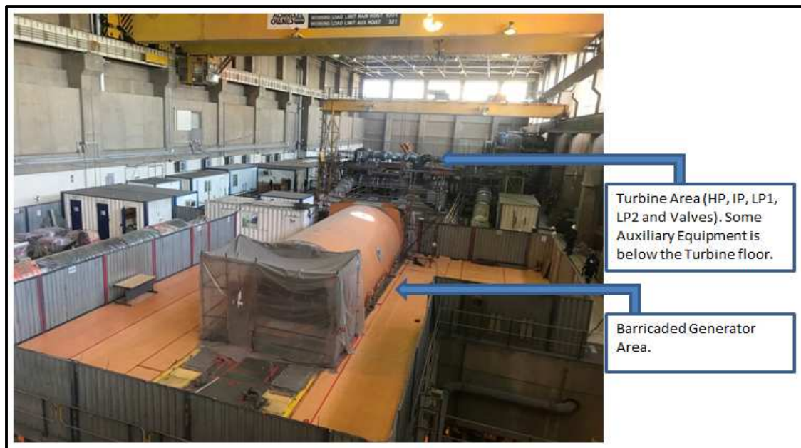
Figure 20: Visual Imagery of the Turbine Floor Level. Turbine Area and Generator area shown.
