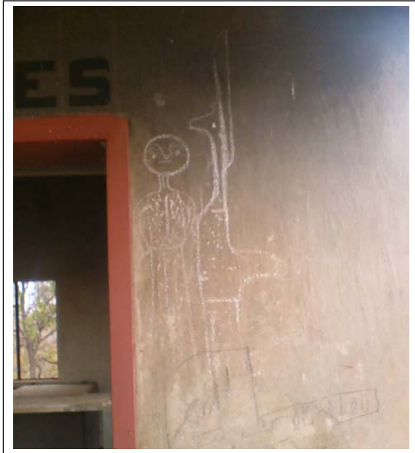
Figure 1.1: Example of graffiti on the walls of the abandoned TEBA buildings in Mozambique.
