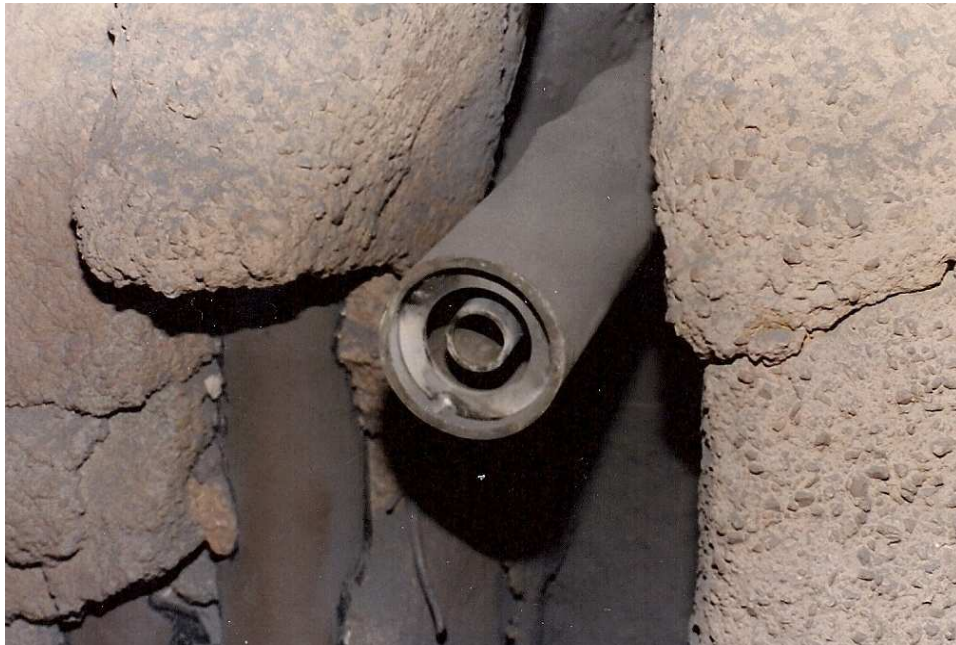
Figure 3.15 Coal slurry nozzle mounted in NFBC wall
