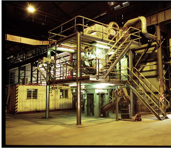
Figure 3.3 The Multi Purpose FBC Pilot Plant
