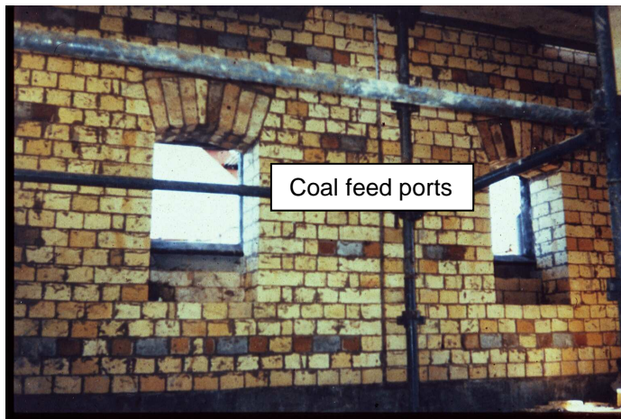
Figure 4.17 Coal feeder wall of the sludge and coal co-fired FBC
