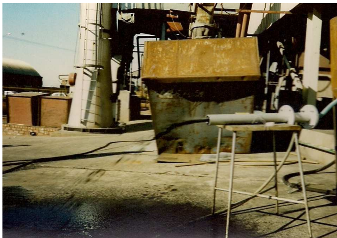
Figure 3.12 Coal slurry injection with increased annular air
