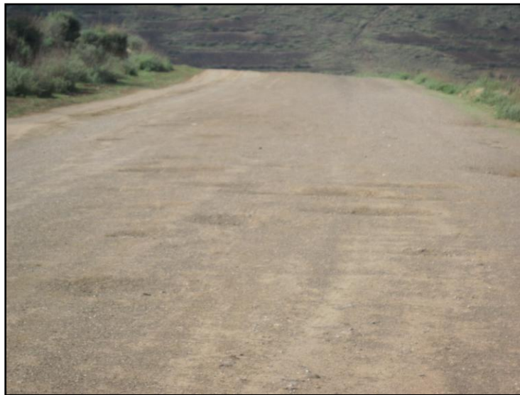
Photo 25: Still unpaved after 25 years since the beginning of the LHWP, the one main road passing Khohlo-Ntso is poorly maintained and filled with deep potholes.
