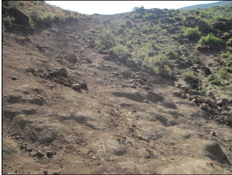
Photo 24: Deep culverts were created by LHWP access roads.
