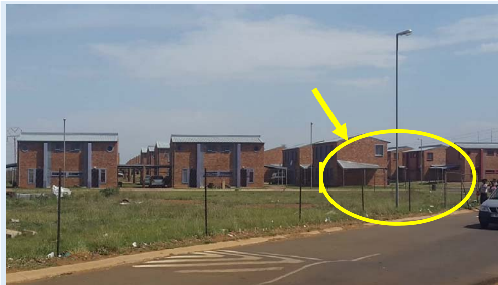
Figure 4.5. Collapsing parking bay roof structure
