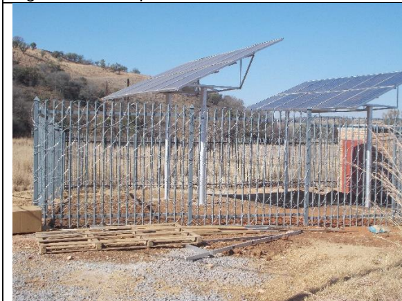
Figure 4.5 : Solar panels powering the borehole
