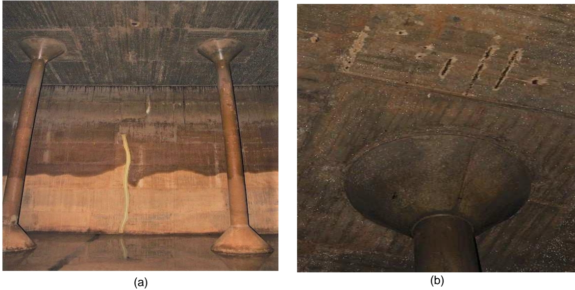
Figure 4.2: Forest Hill reservoir: a) moisture effects on wall b) corrosion on roof slab
