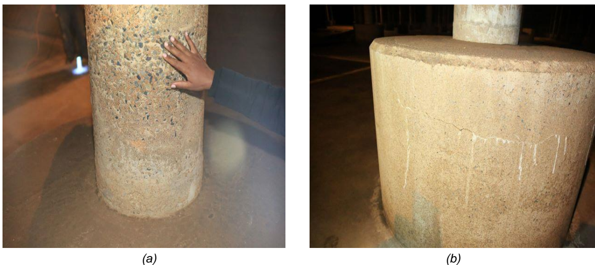
Figure 4.3: Brakfontein reservoir: a) exposed aggregate on column inside, b) cracked base leaching
