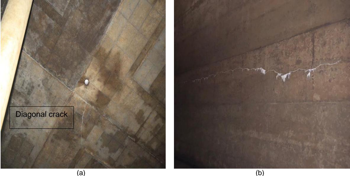
Figure 4.1: a) Roof cracked and leaching for Forest Hill reservoir b) Internal wall leaching for Forest Hill reservoir
