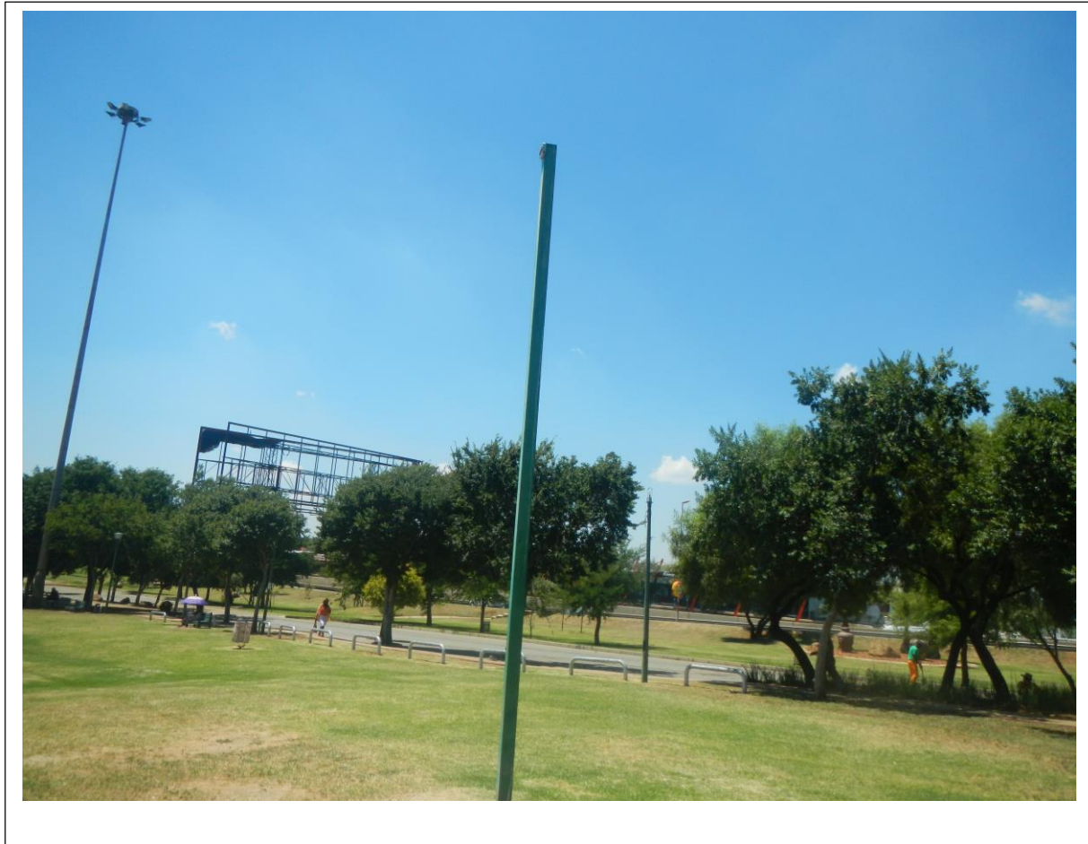
Figure 4.9: Dysfunctional lighting at Thokoza Park (foreground) and a functional lighting (background) (enlarged photo of number 3 in figure 4.2)
