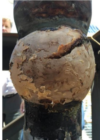
Figure 3.10. Damaged putty due to fault current surge. (Courtesy of Patrick O'Holloran)
