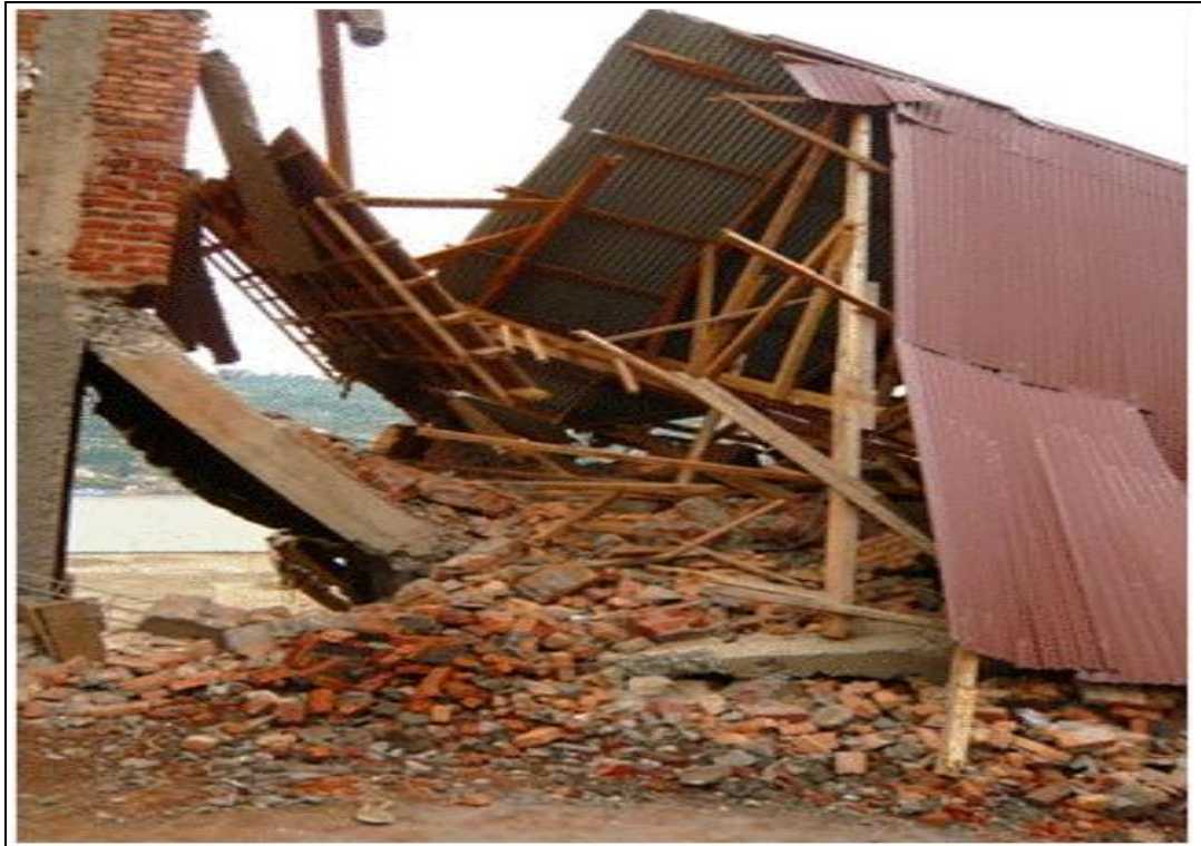
Figure 1.2 Damage to a house resulting from earthquake on 3/2/2008 at Bukavu City (D.R Congo). Source: I. Badriyo, Project UNOPS “Unite de gestion de risques volcaniques”, Goma, North-Kivu, Democratic Republic of Congo
