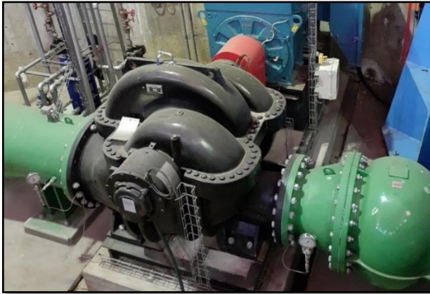
Figure 2-8: Photograph of a centrifugal pump at the DWS Nottingham Pump Station in the Northern Cape
