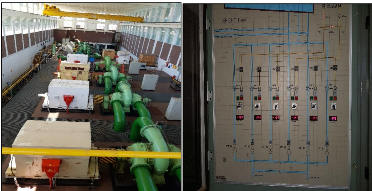
Figure 4-3: Photographs of Jericho pump station equipment.
