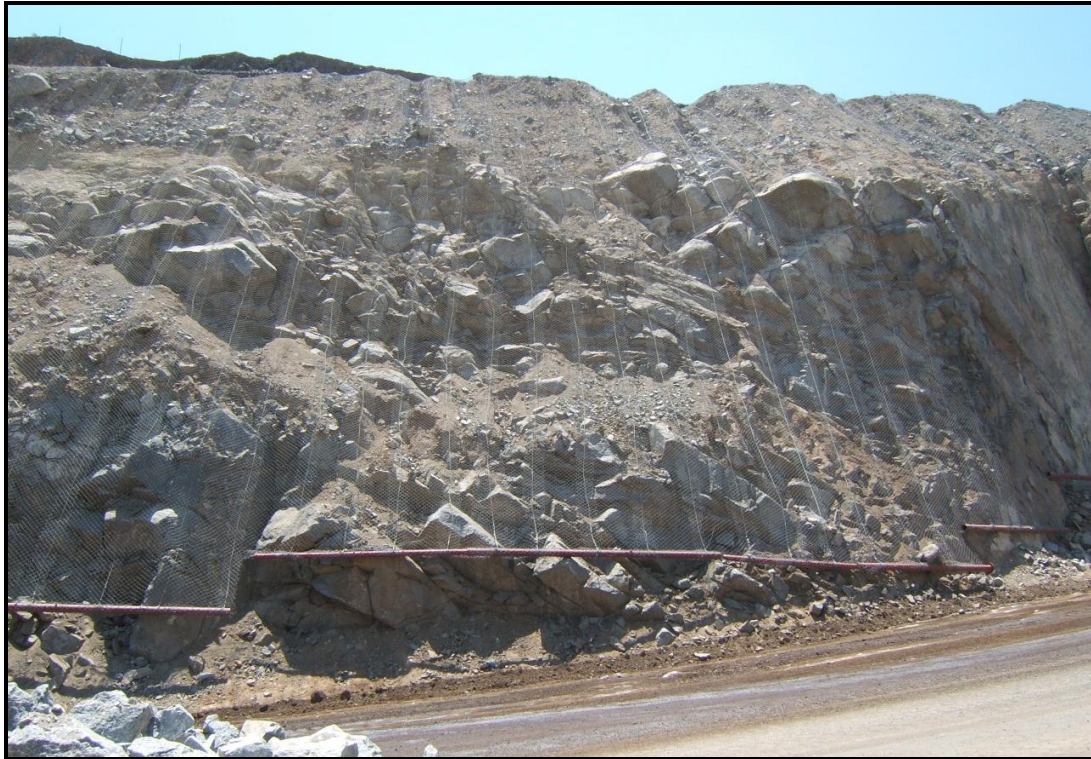
Figure 8.18 Wire meshing to reduce the rockfall hazard
