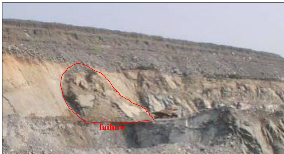
Figure 9.16 Photograph taken by the radar of a stack failure on the west wall
