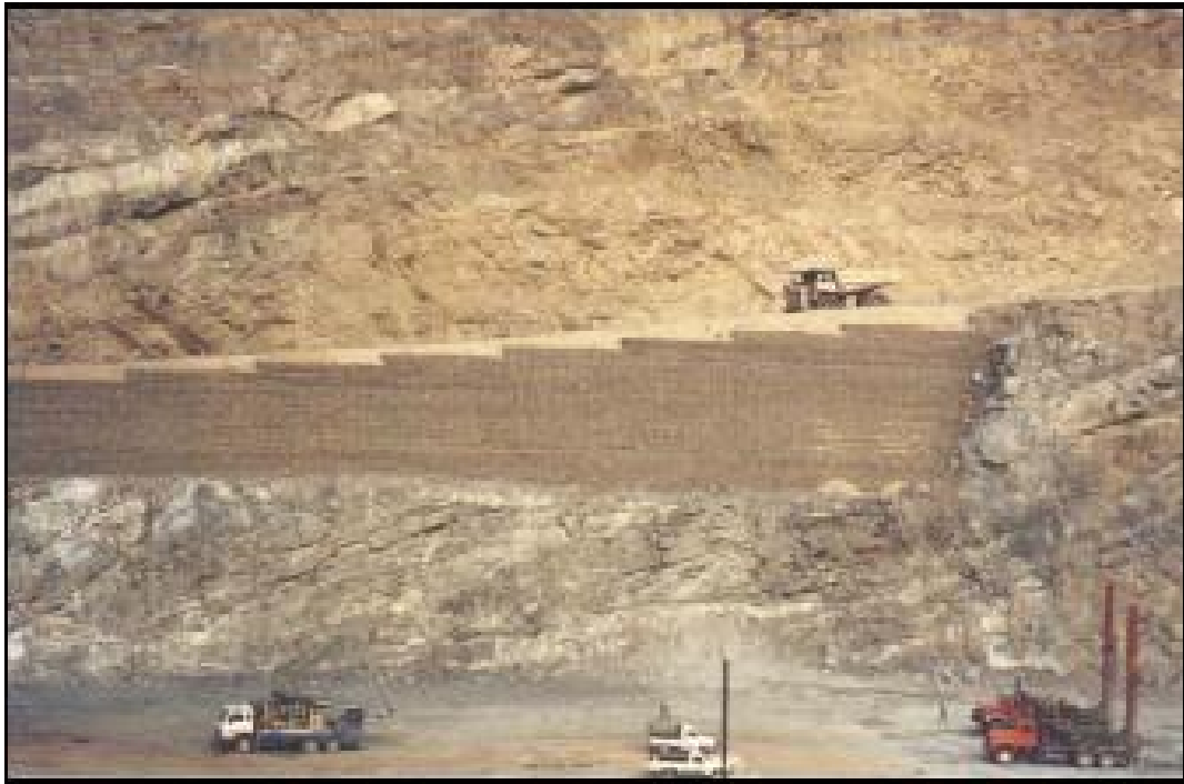
Figure 8.16 Gabion wall supporting the backfilled footwall ramp in Sandsloot (Bye and Rorke, 2002)
