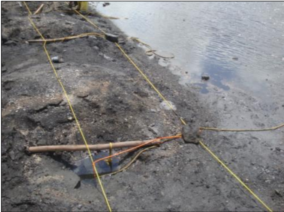
Figure 12: Pre-split tie-up on surface with a single charge suspended into the blast hole (Photo taken by Marton, 2010)
