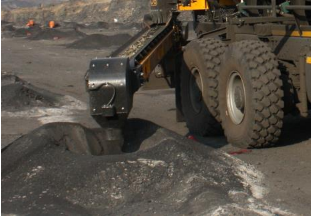
Figure 30: Stemming truck conveyor delivering stemming material into the blast hole (photograph taken by Botha, 2011)
