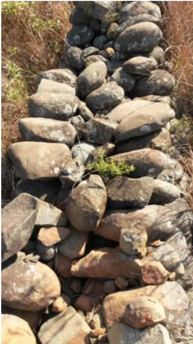
Figure 4.11: Photograph illustrating the method of construction used for building walls(Photograph Tiffany Henshall)
