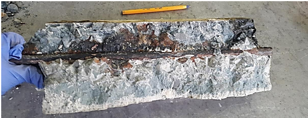
Figure 3.8: Photograph showing corrosion products within the concrete cover depth
