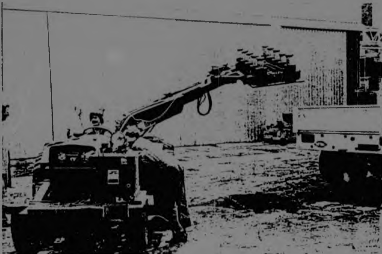
Fig. 22—The self-propelled jacking unit designed and built for the pre-compression of reinforced wall
