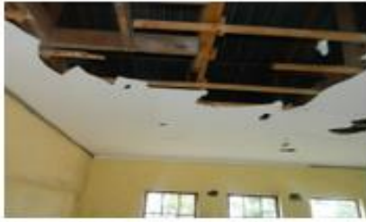
Image 1. Dangerous building structure
